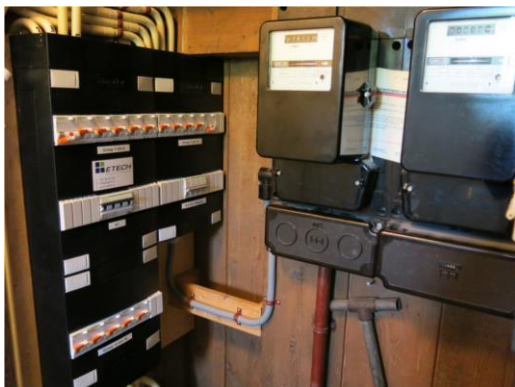
kWh-meter Dorpskerk (linker kWh-meter)
